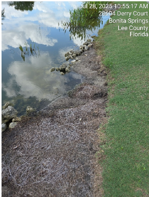
Lake 6A - Erosion needs repair.
