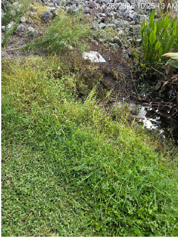
Lake 16 – Gully needs repair.
