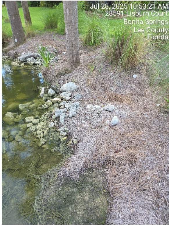
Lake 6A – Erosion needs repair.
